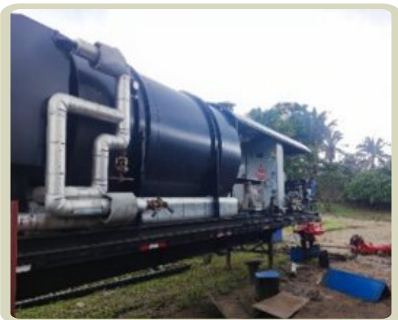
ON-SITE STEAM GENERATOR
